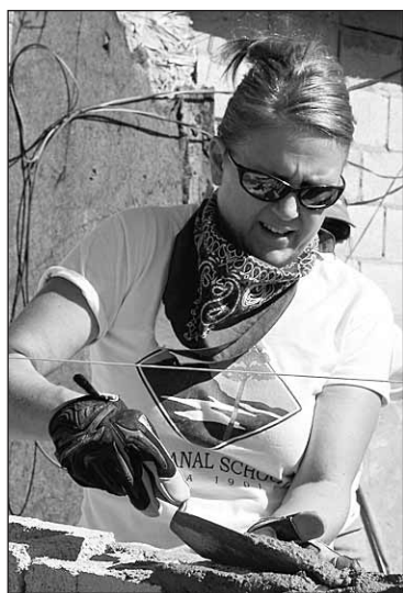
Suncreek UMC's Deniece Mason lays mortar for a new cinderblock home in a suburb outside of Ciudad Juárez, Mexico.
